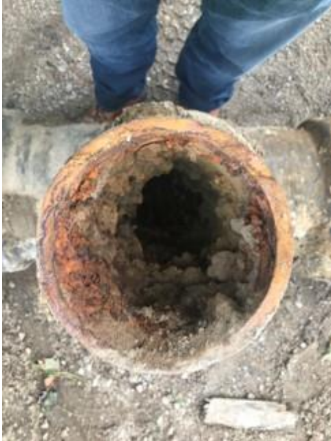
Typical Old Un-Lined Cast Iron Pipe
