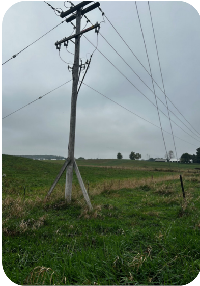
Swamp shoes were installed on transmission poles through wetlands to provide power to McLaren Greater Lansing Hospital.
