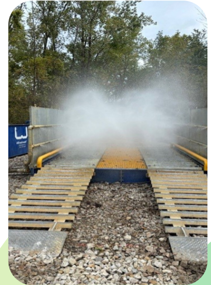
A wash station was installed for construction vehicles to remove invasive species before entering the wetland area.
